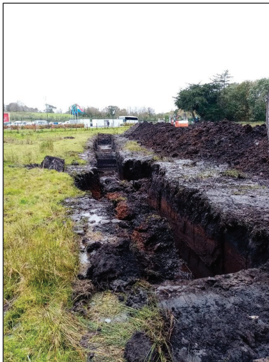
Plate 5 Trench collapse at north-eastern end of Test Trench 1
