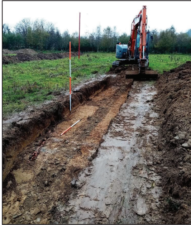
Plate 27 Trench 31 with linear band of redeposited soil representing cut and fill (Context 25) for stone lined culvert
