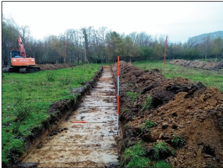
Plate 26 Trench 34 with Trench 33 to right and Trench 35 being excavated to left of photo
