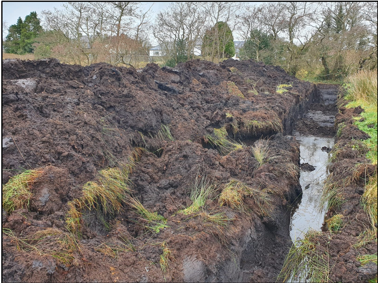
Plate 3 Collapse in Trench 5.
