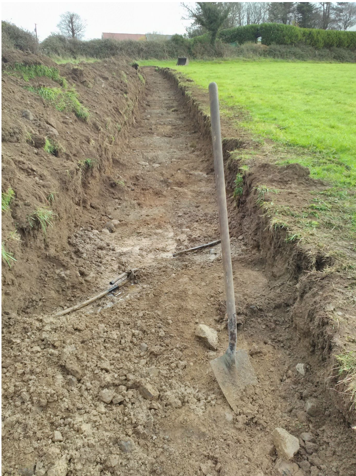
Plate 2 Excavation of Test Trench Two showing gravel (Context 3) and clay (Context 1) and marl (Context 2) above it
