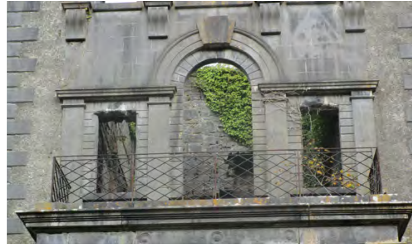
Potential for re-roofing and redevelopment of the balcony above the main entrance door
